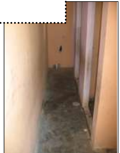
The bathrooms are unsanitary
